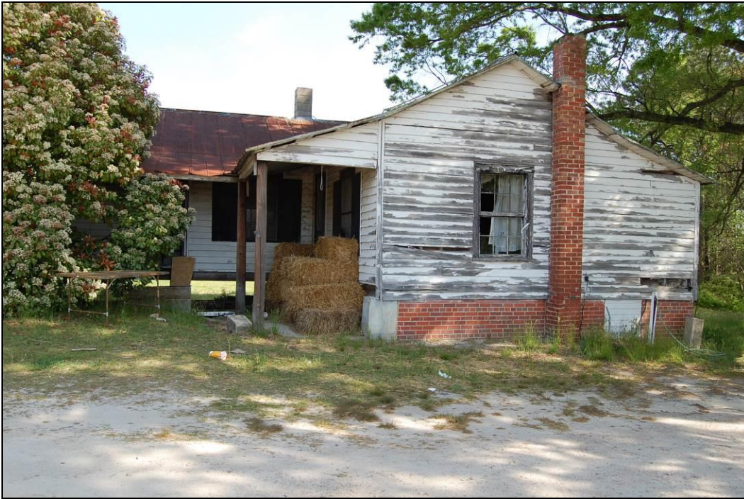
Figure 43. South side and west front elevations of house; note loss of porch floor and posts
