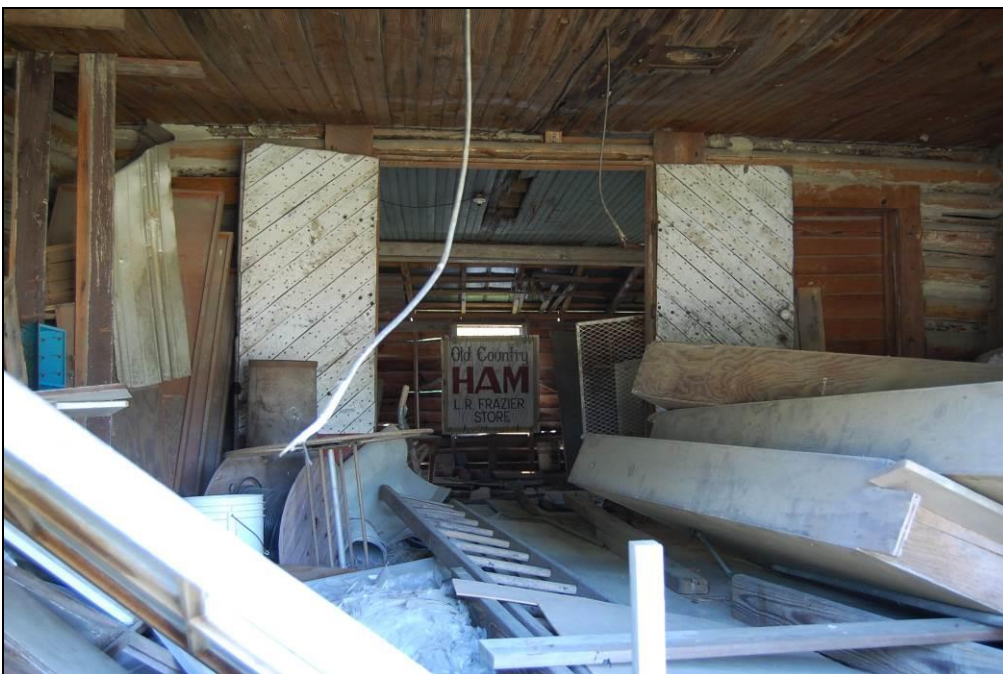
Figure 32. Interior of log section of store viewed from opening at north gable end
