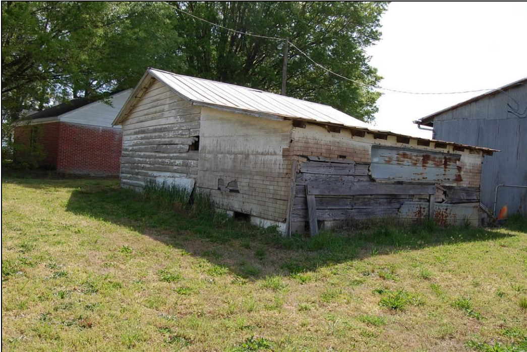
Figure 16. Shed [4] at center, garage [2] at left, and tractor shed [5] at right, looking southeast
