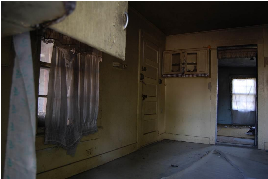
Figure 45. Looking into kitchen through window located adjacent to flue stack at south side elevation of house
