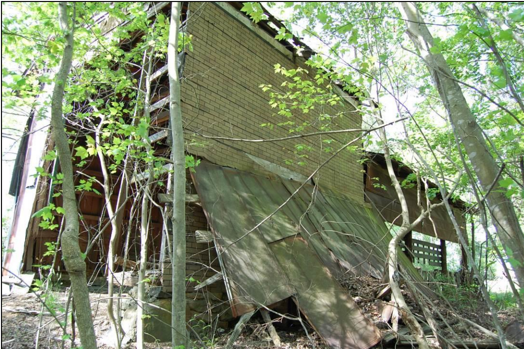
Figure 50. Looking southwest at tobacco barn, with wall removed at left, and tractor shed at right
