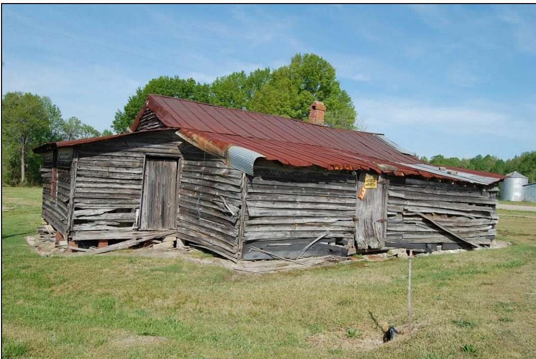
Figure 34. South gable-end and east side elevation of store, displaying both shed additions.
